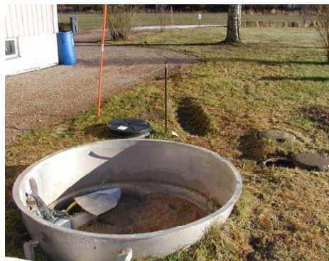
Fig. 2. Filter well for a single house using the material Polonite.
